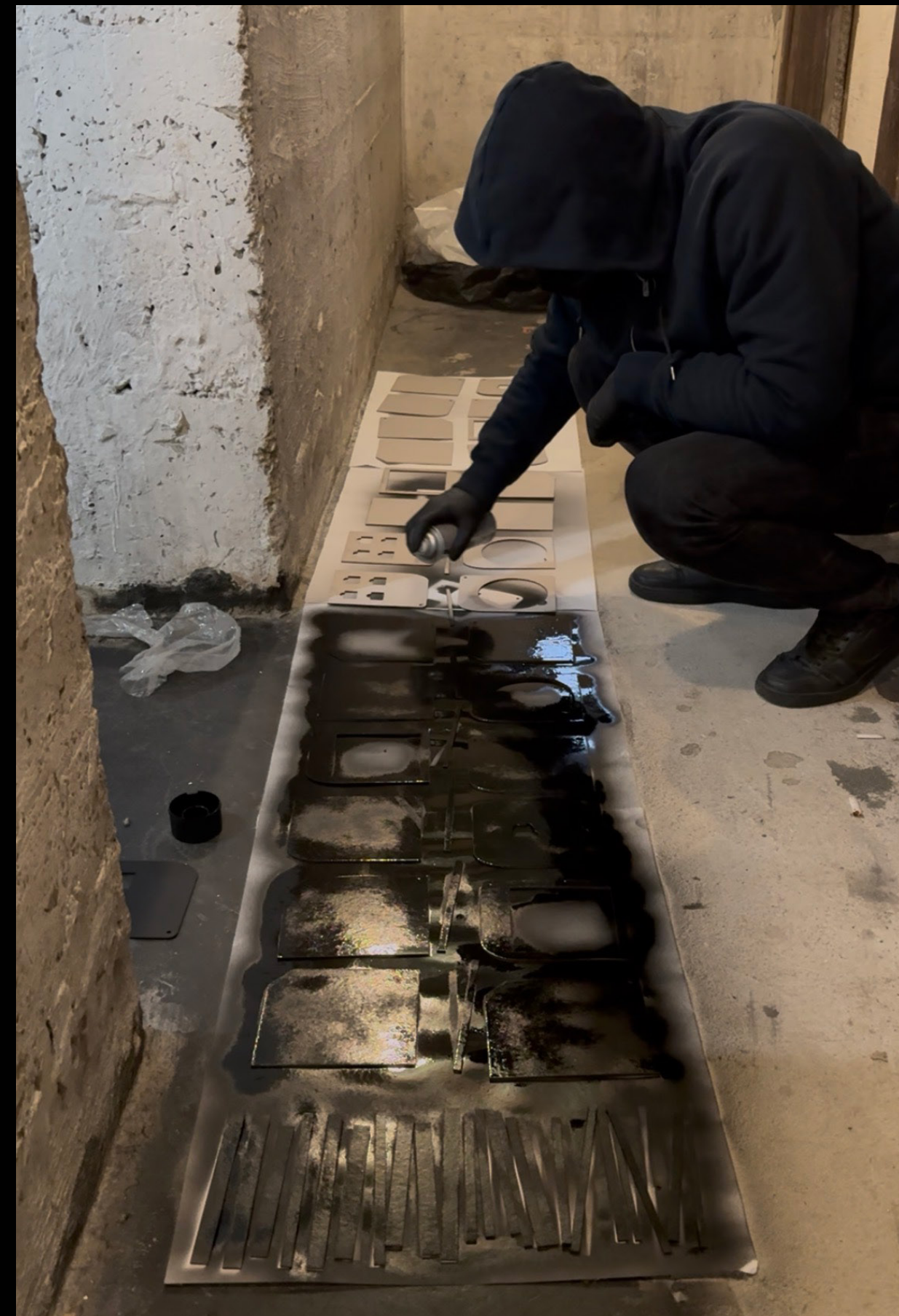
After all pieces had been cut, the components were laid out and finished with a matte black spray paint coating to achieve a cohesive appearance.
